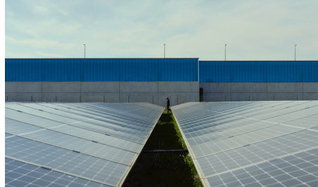
Solar park in Belgian plant
